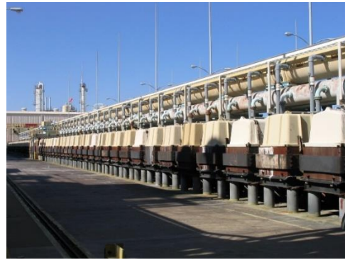
Figure 3. Chlor-alkali cell line with MDC-55 diaphragm cells 15
